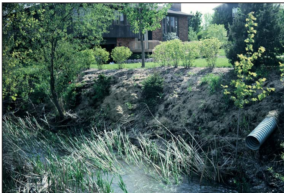
Underneath the lawn clippings is an exposed streambank. Invasive plants like the buckthorn shrub (near the pipe) and reed canary grass (in the water) offer no stabilizing roots to stabilize the bank. These invasive plants should be removed and replaced with native vegetation.
