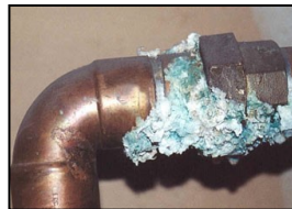
Drinking water pipes with visible copper corrosion.
